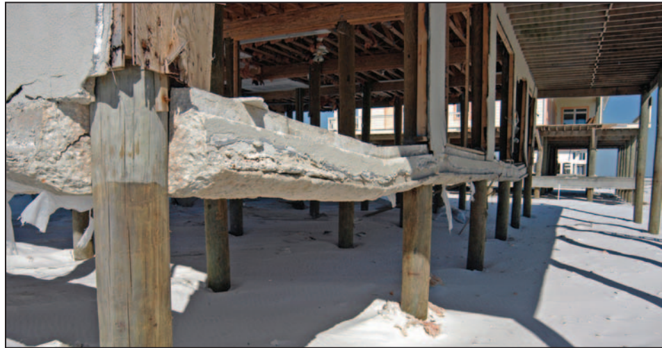
Figure 3-25. The sand underneath this Pensacola Beach, FL, building was eroded due to wave runup and storm surge (Hurricane Ivan, 2004)
