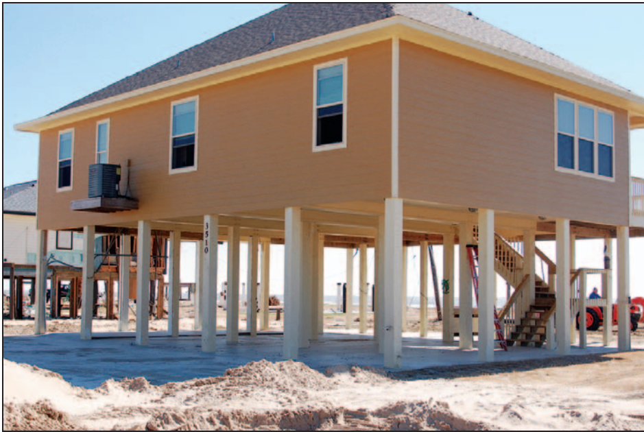
Figure 2-19. Breakaway walls below the first floor of this house broke as intended under the flood forces of Hurricane Ike (Bolivar Peninsula, TX, 2008)
