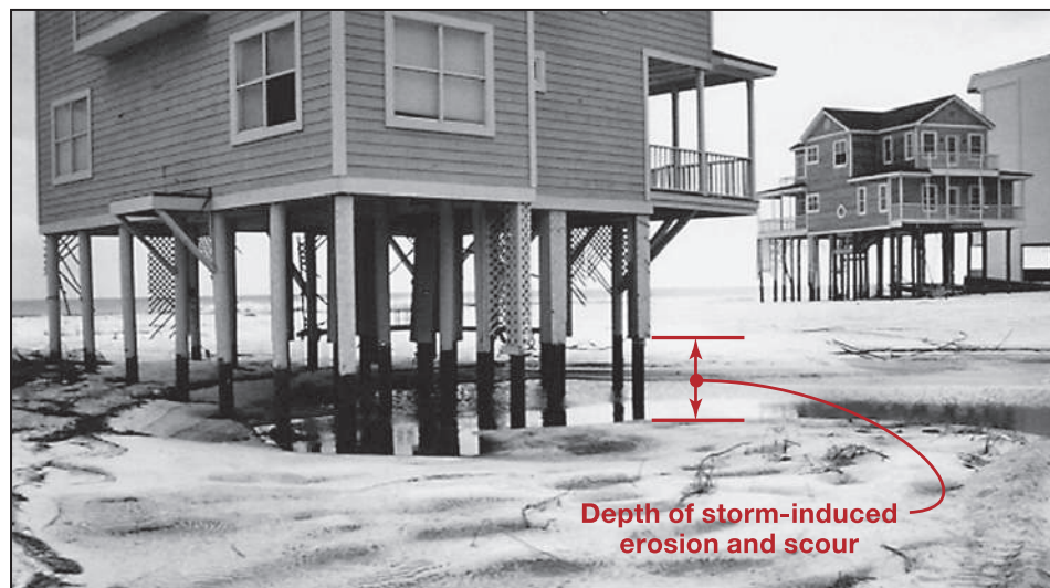
Figure 3-21. Pile-supported house in the area of channeled flow shown in Figure 3-20. The building foundation and elevation successfully prevented high-velocity flow, erosion, and scour from destroying this building
