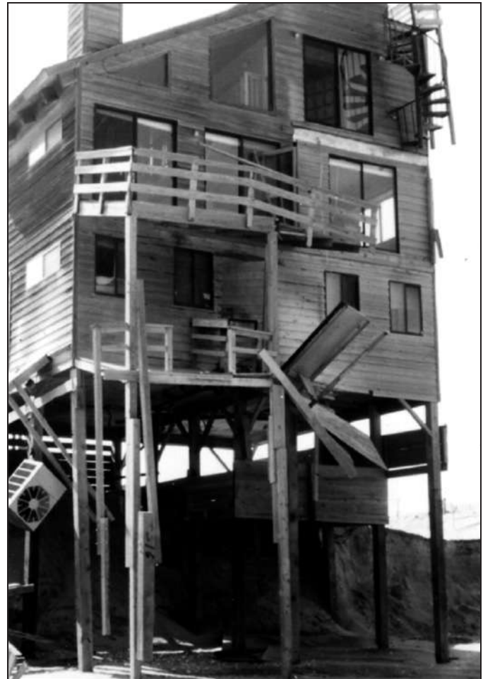
Figure 2-3. Although this house seems to have lost only several decks and a porch during the March 1989 nor'easter, the loss of supporting soil due to long-term erosion left its structural integrity in question following successive storms
